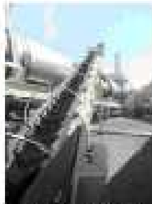
Photo 2b: Conveyor belt for RAP at the TBM 25 at the ACC work site at La Ferté Macé
