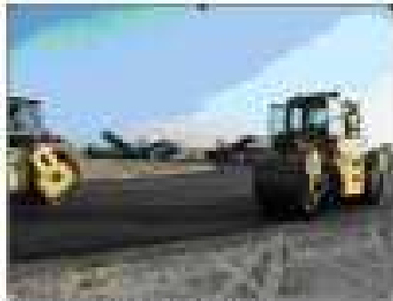
Photo 1a: Laying the layer of WMA (hot bitumen + RAP) with 20% of RAP at La Ferté Macé
