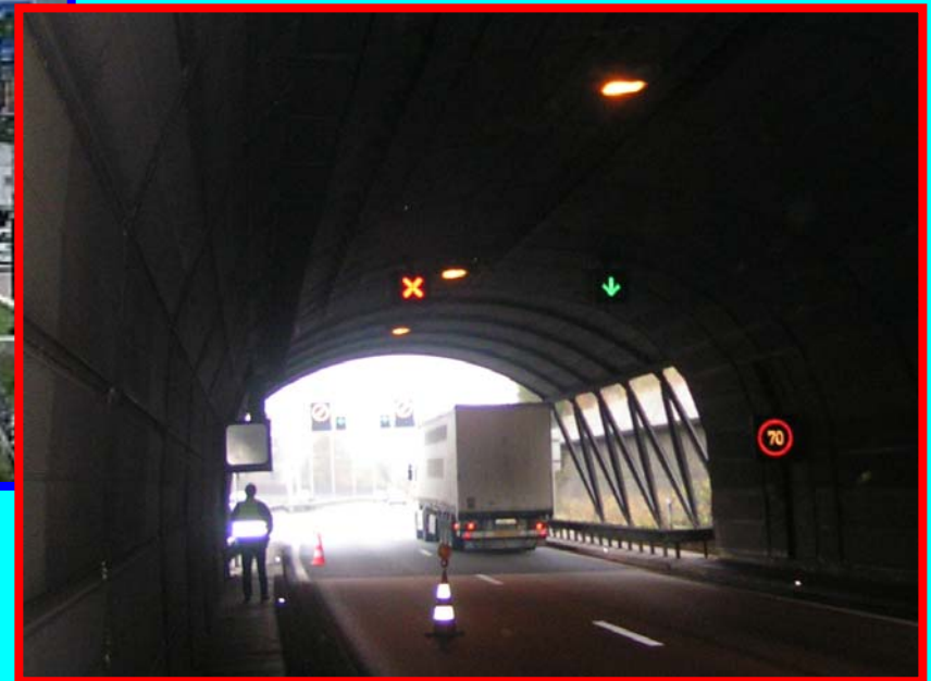
VMS Lane signing
